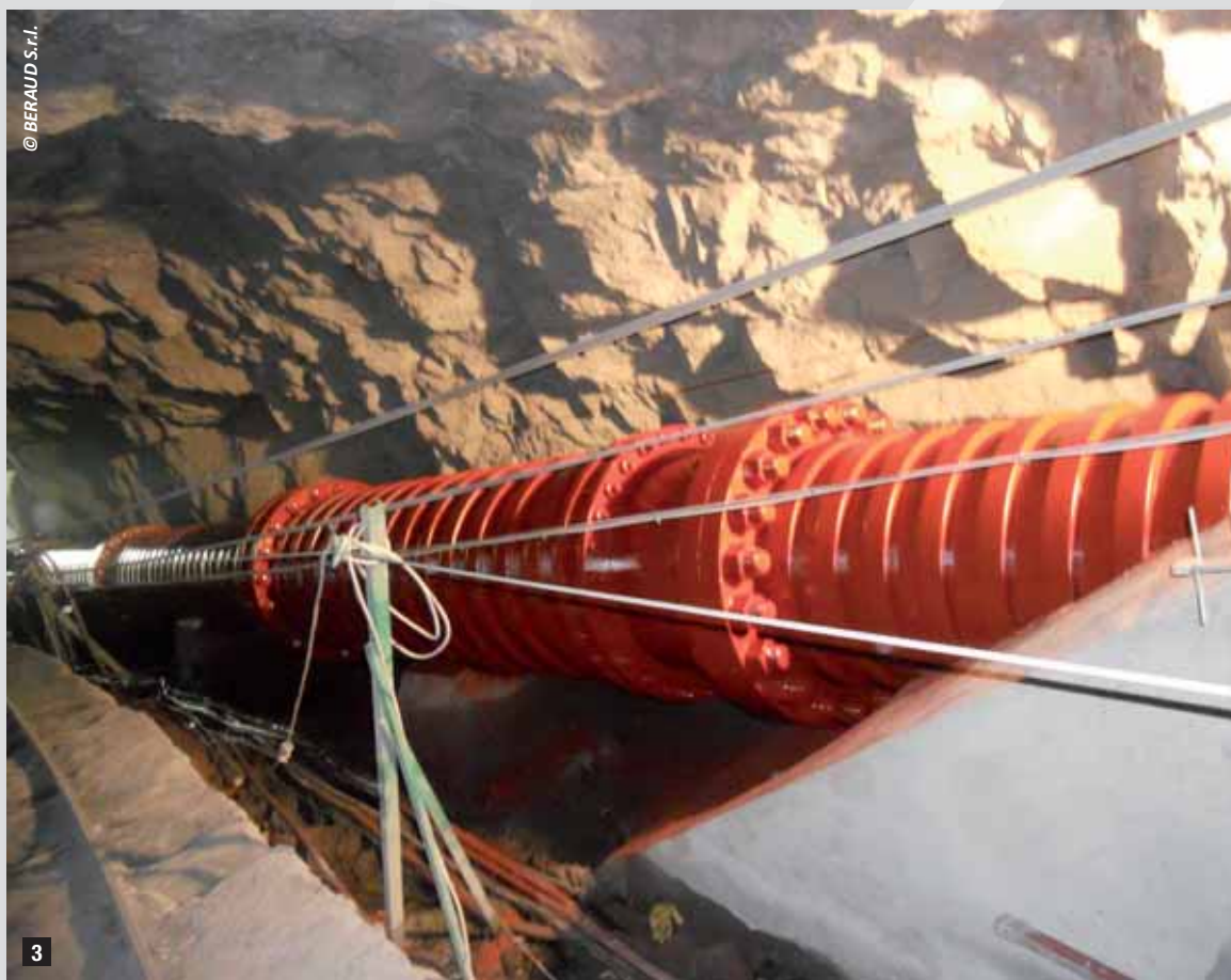
3 The maintenance operations aimed at restoring the external and internal protection of the pipeline, carried out in July, August, and September 2013.
